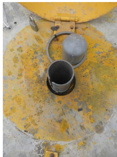
量測導管俯視
