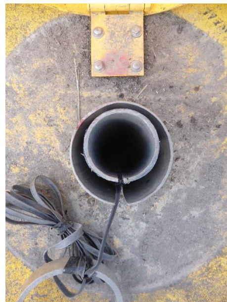
量測導管俯視
