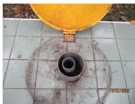
量測導管俯視
