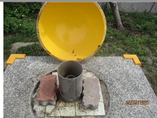
量測導管俯視
