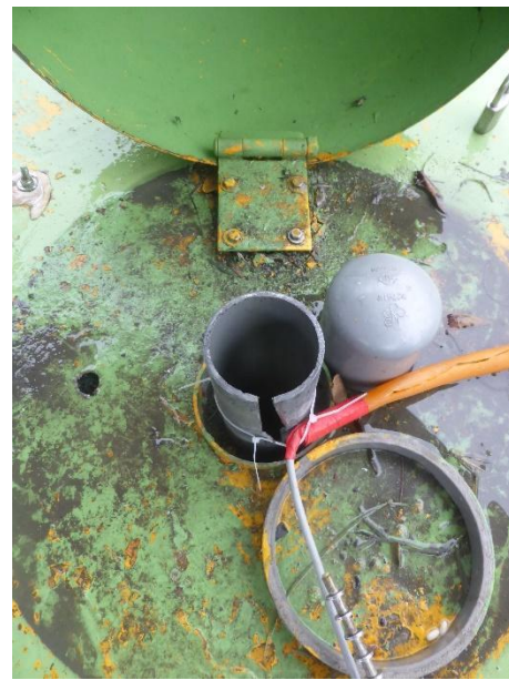
量測導管俯視
