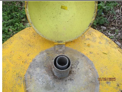
量測導管俯視
