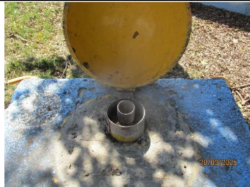
量測導管俯視
