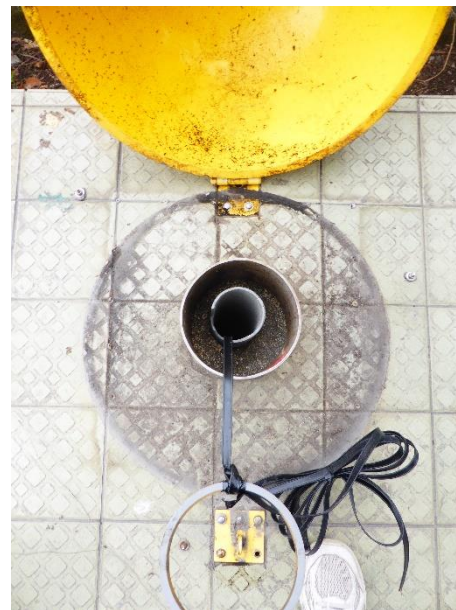
量測導管俯視
